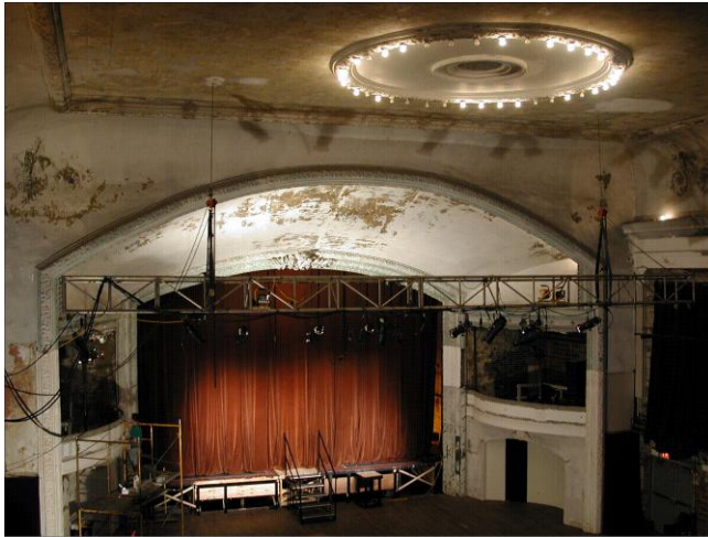
Capitol Theatre had chipped paint and plaster falling off the walls.
